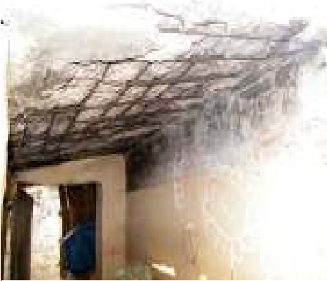
A degraded RCC ceiling. People neither have the money nor the skill and knowledge to maintain and repair these kind of structures. Chatar Ghat, Khagaria District, Bihar.
