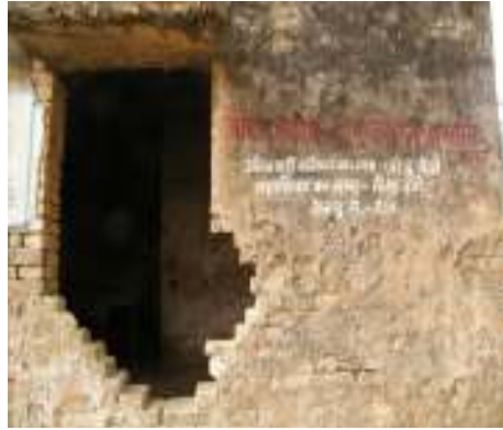
An Indira Awas Yojana structure which is degraded and dangerously falling apart being used as an Anganwadi. People are not able to maintain it, but continue using this structure. Ilmas Village, Samasthipur District, Bihar
