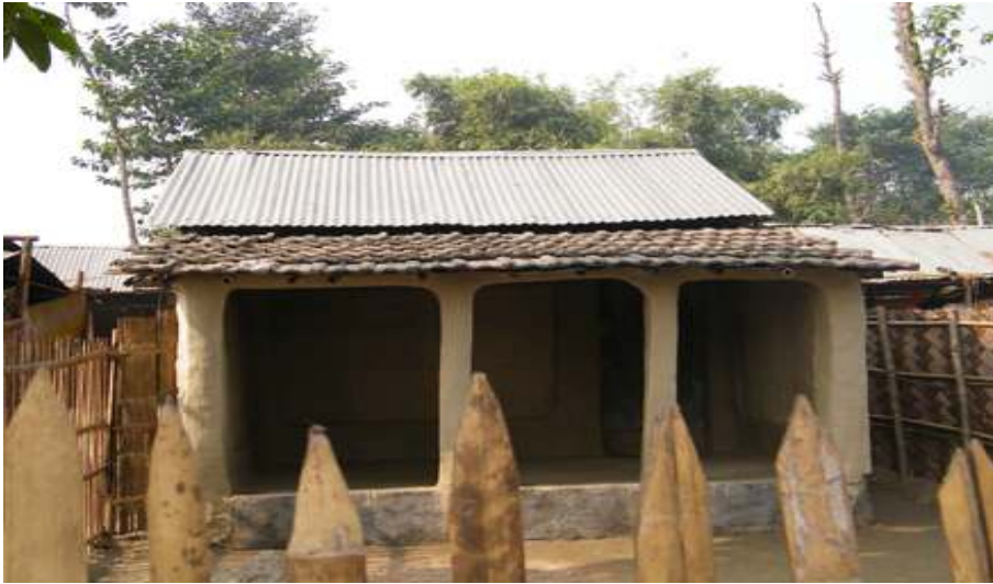
A fusion house: tile-roof verandah; GI-sheet roof for main house, mud walls, bamboo roof structure. A lot of the materials are recycled materials retrieved from the old damaged house.
