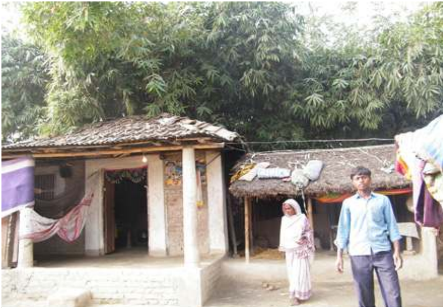
An Indira Awas Yojana house of brick and cement, tile with bamboo roof structure, cement columns and a mud-thatch-bamboo sleeping quarters as an additional room. - Jorgama, Madhepura District, Bihar
