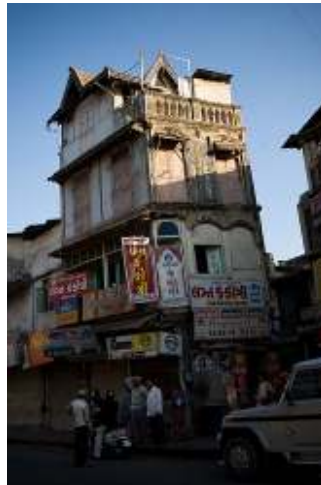
Figure 1: A leaning building. Recipe for disaster.
